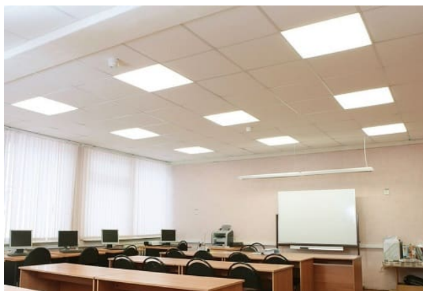
Figure 19 - LED panels for lighting classrooms and laboratories
